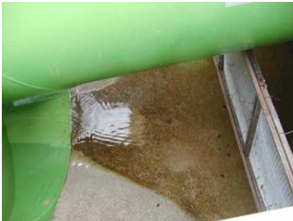
Figure 6. Intake with fish screens
